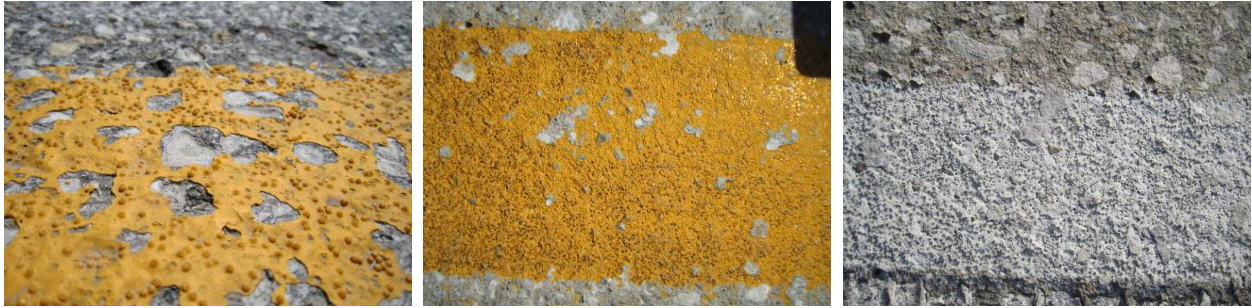
Figure 15. Material loss on paint products after two winters
