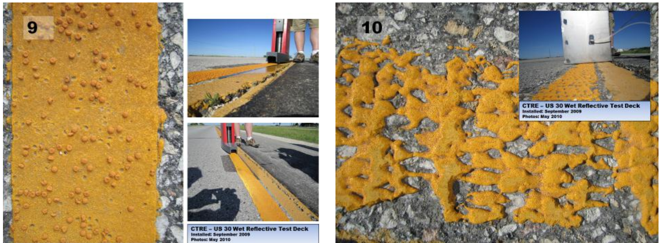
Figure 10. Ennis test sections 9 and 10 after one winter
