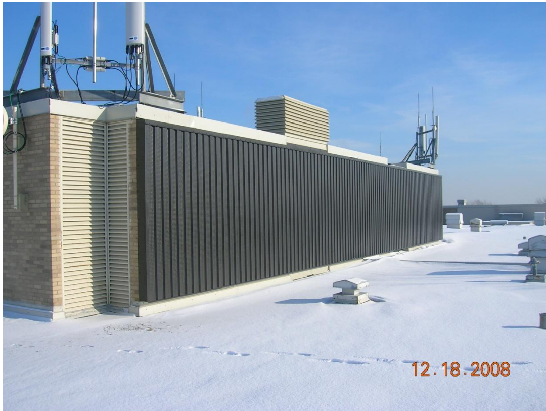
Figure 1.1.15: Solar wall installation at St. Anthony Village High School (Source: Bernie Eikmeier, MnKinstry Co.).
