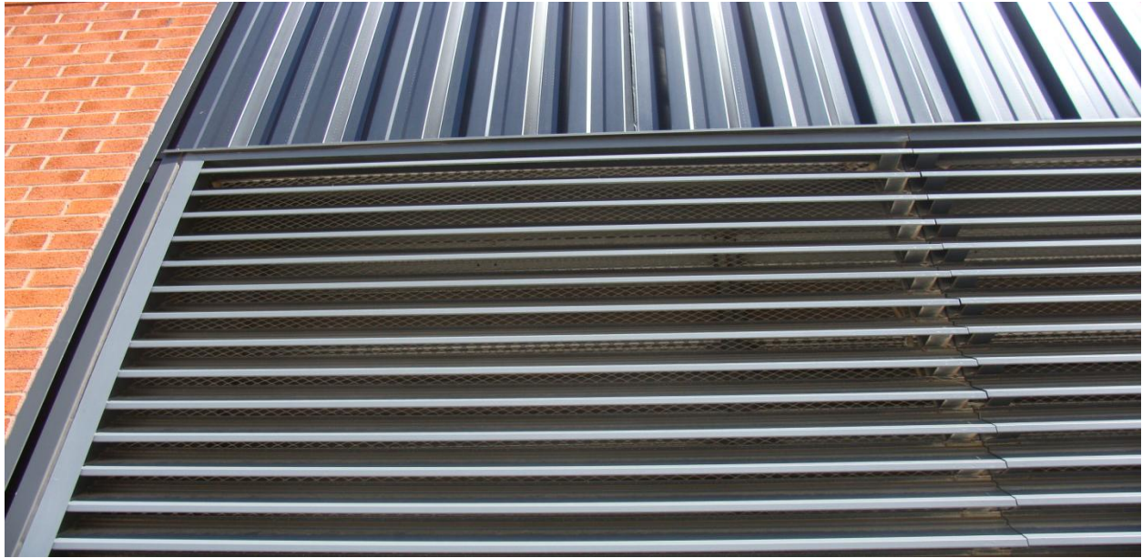
Figure 1.1.13: Close-up of IDDS bypass air entry.
