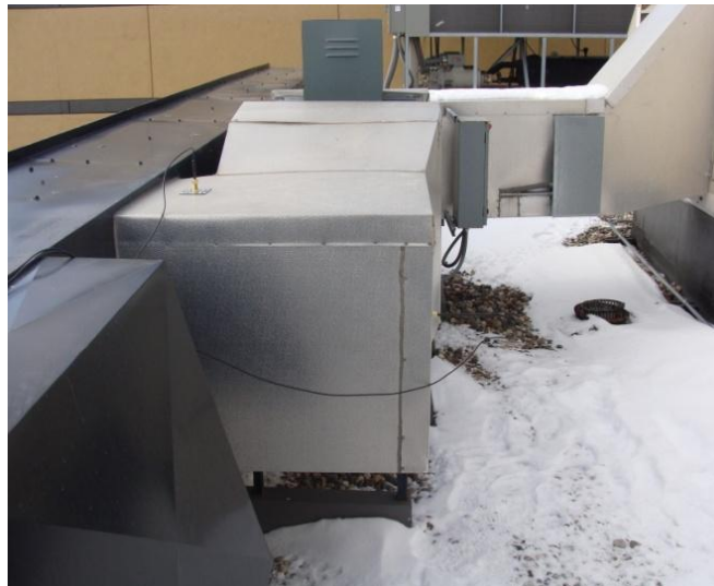
Figure 12: Close-up of both installed temperature sensors at 3 rd Precinct (one on top and one on side).
