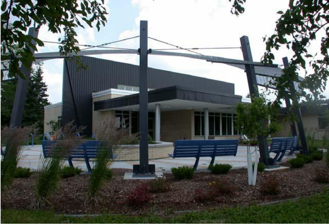
Figure 1.1.16: Solar wall installation at Hibbing Courthouse front view (Source: Conservall case study.).
