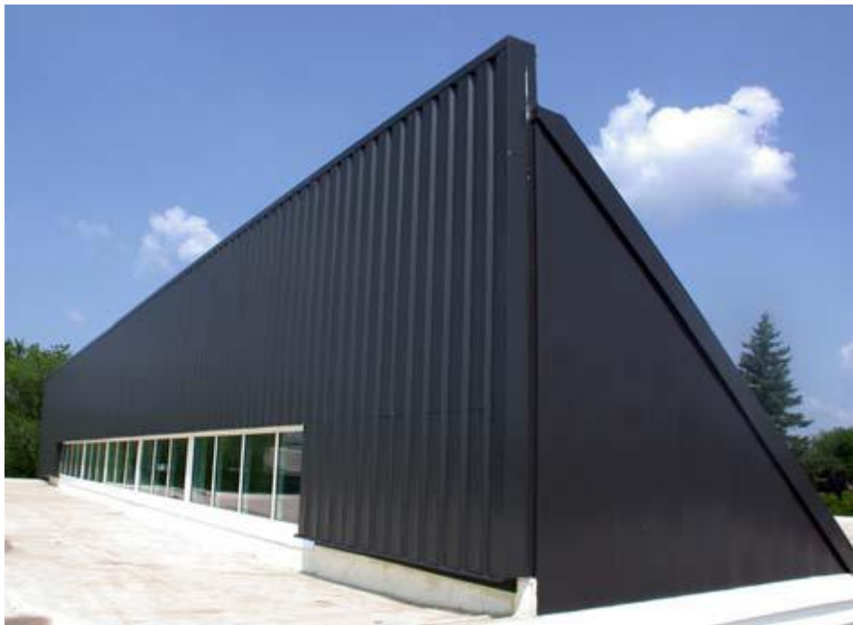
Figure 1.1.17: Solar wall installation at Hibbing Courthouse 2 nd elevation (Source: Conservall case study.).
