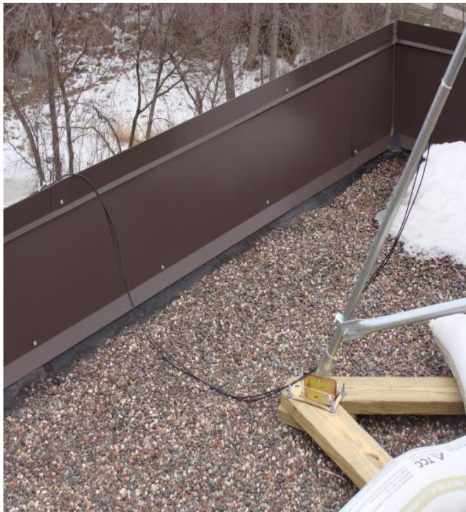
Figure 17: Temperature sensor wiring leading to the weather station.
