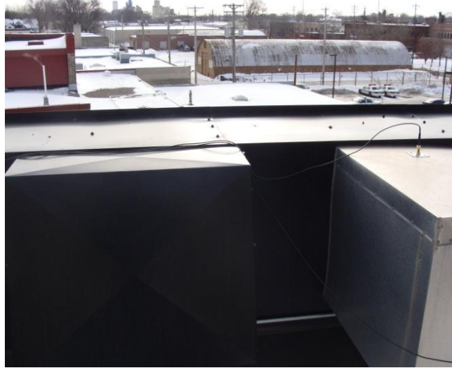
Figure 13: Routing of sensor wires over ductwork.
