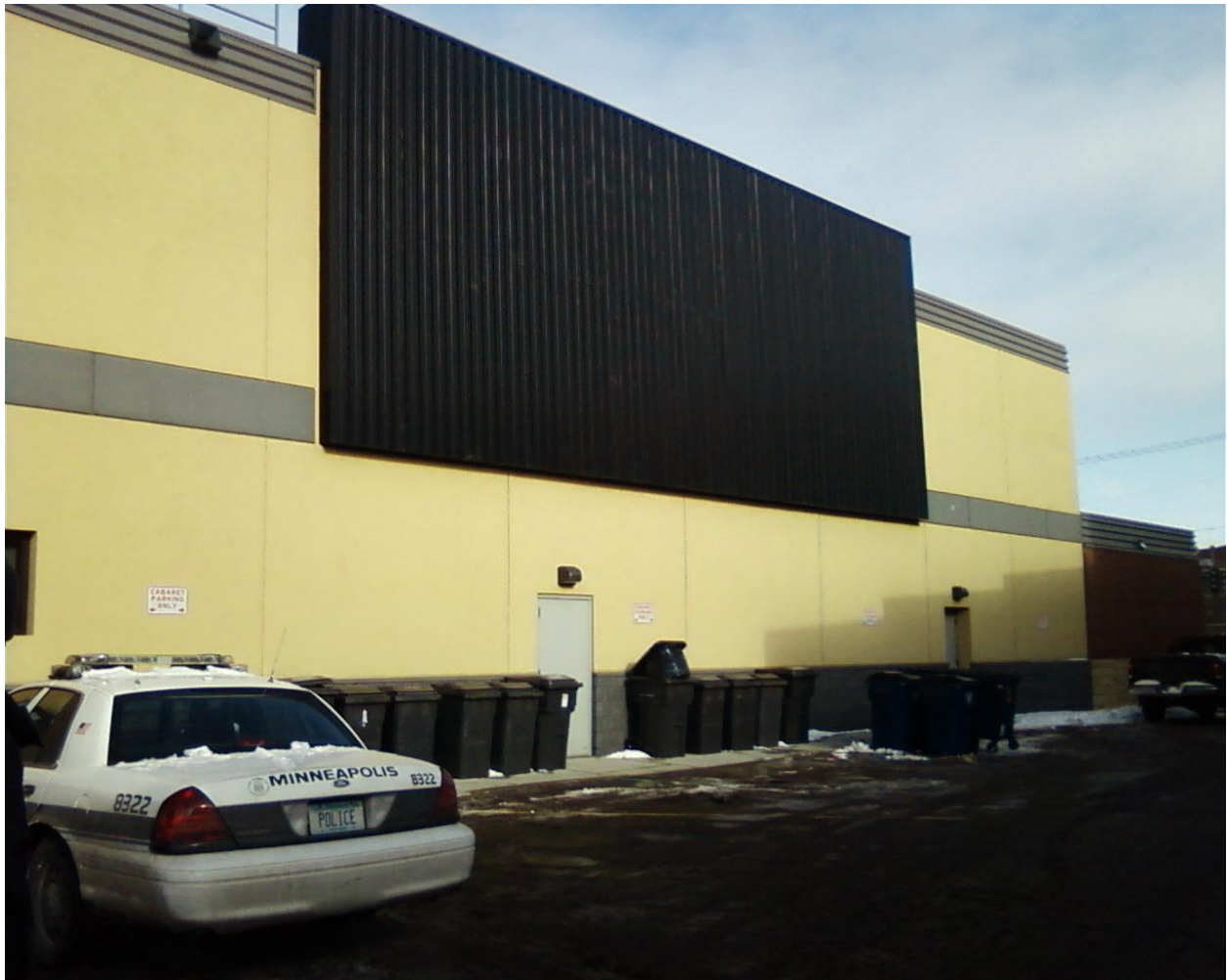
Figure 1.1.5: Solar wall installation at 3 rd Precinct Police station.
