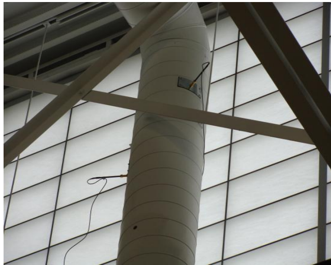
Figure 15: Air duct temperature sensors installed at the Breck School.
