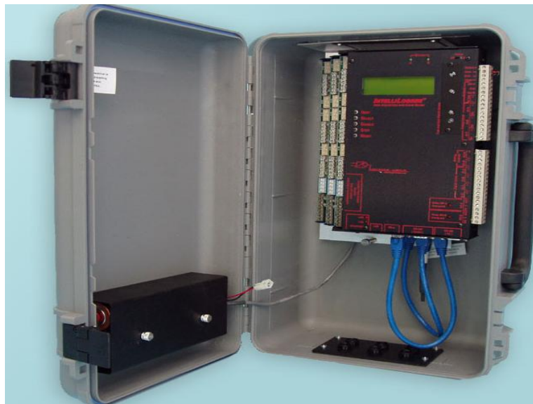
Figure 19: IntelliLogger data logger used for the wall profile measurements at the Breck School.
