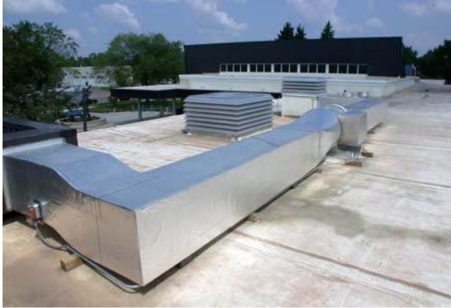
Figure 1.1.18: Hibbing solar wall ducting on roof (Source: Conserval case study.).
