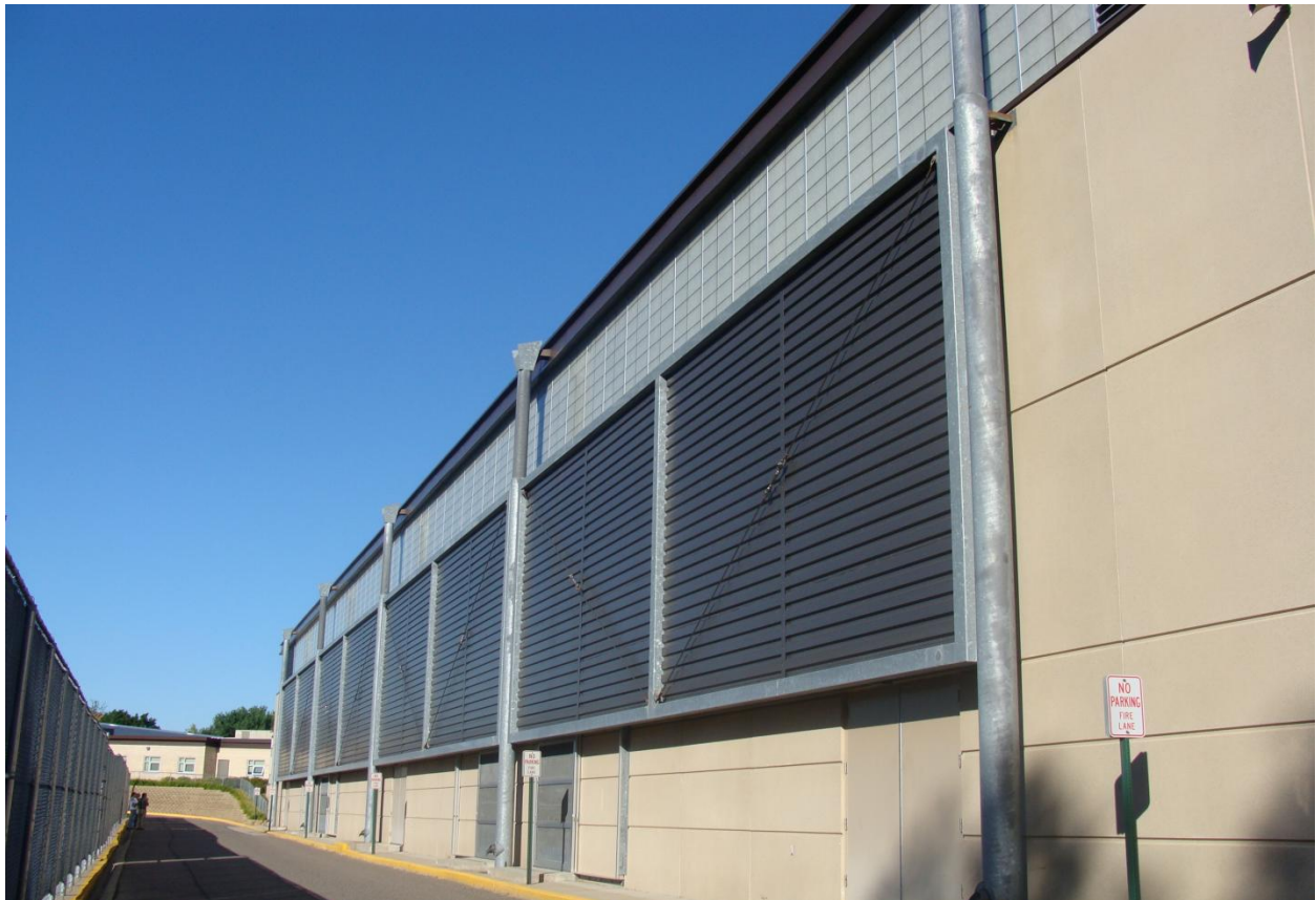
Figure 1.1.1: Solar wall installation on Breck School gymnasium wall.
