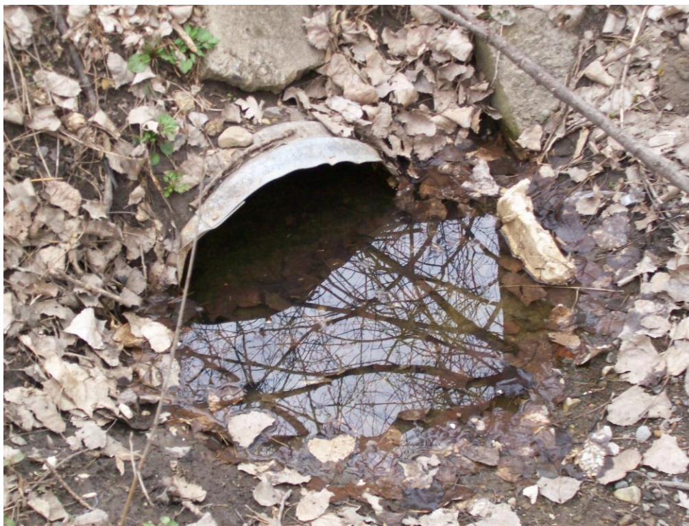
Figure 24. Drainpipe confirmed by MPCA to be running from internal drains of former Year-A-Round Cab Company into US-14 Ditch with sheening and discoloration.
