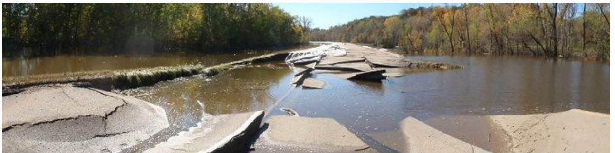
Figure 1.3: US Highway 169 south of St. Peter, Minnesota after Minnesota River flooding in fall 2010 (Unknown, 2010)
