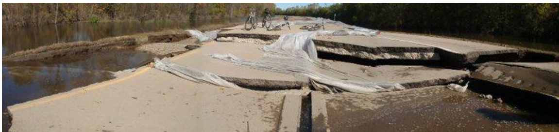
Figure 2.2: Highway 169 north of Mankato, MN after flooding in October 2010 (Unknown, 2010)
