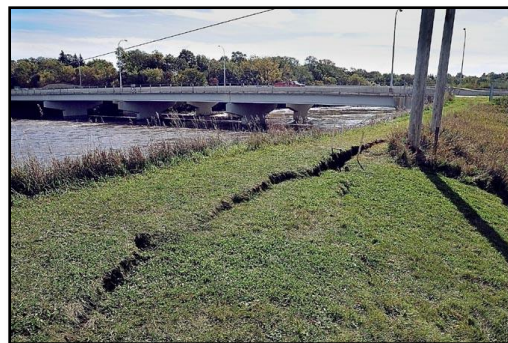
Figure 1.1: Mankato Levee Damage September 2010 (Linehan, 2010)
